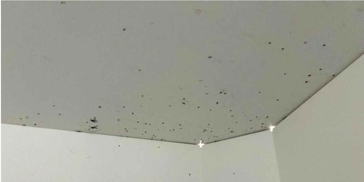
Figure 22. Insect Infestation in Shower Facilities; Observed January 21, 2026
